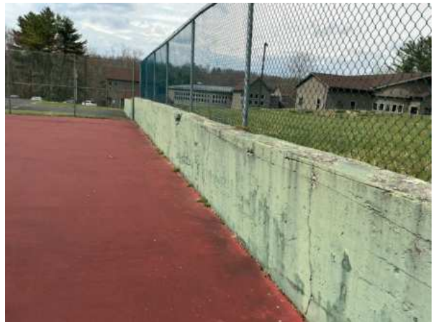
Cracks and deterioration
