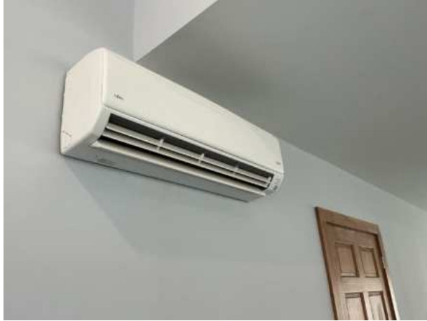
Mini-split air handling units at the Entertainium building
