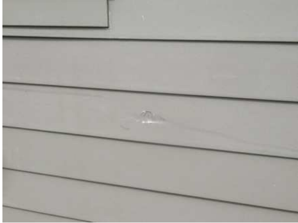
Damaged siding at the clubhouse
