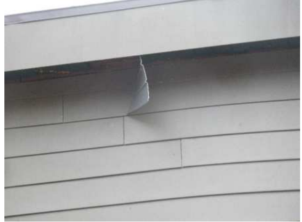
Loose trim at the entertainium building
