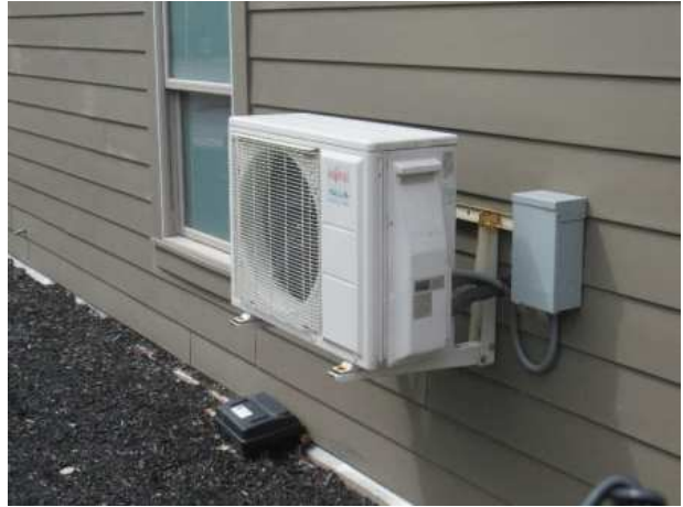
Mini-split condensing units at the pool house
