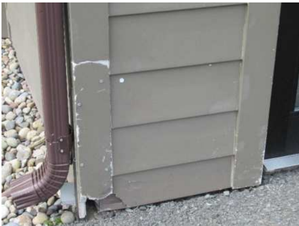
Damaged siding and trim at the clubhouse
