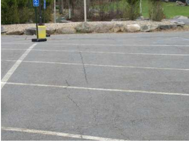
Cracks at the pool house parking area
