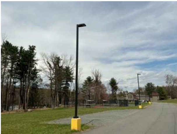
Light poles and fixtures at the main entrance way
