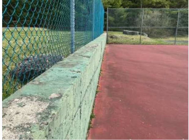
Leaning section and deterioration
