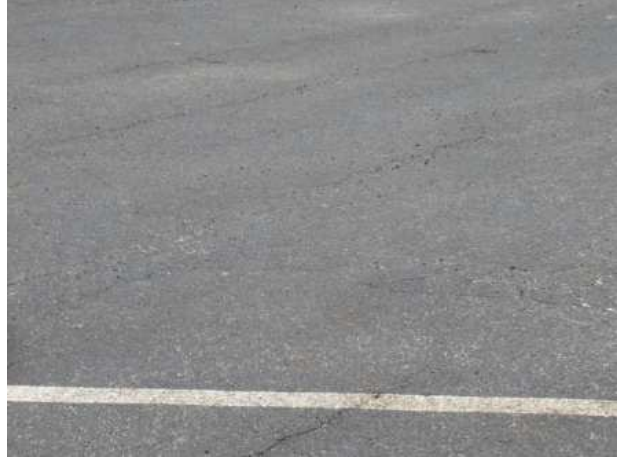
Cracks at the pool house parking area
