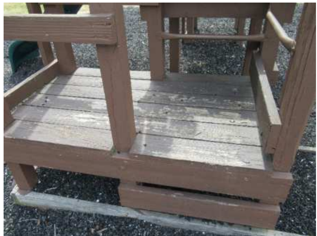
Weathered wood components
