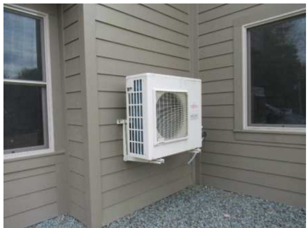
Mini-split condensing units at the Entertainium building
