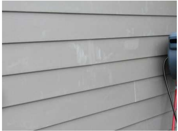
Paint finish deterioration at the pool house
