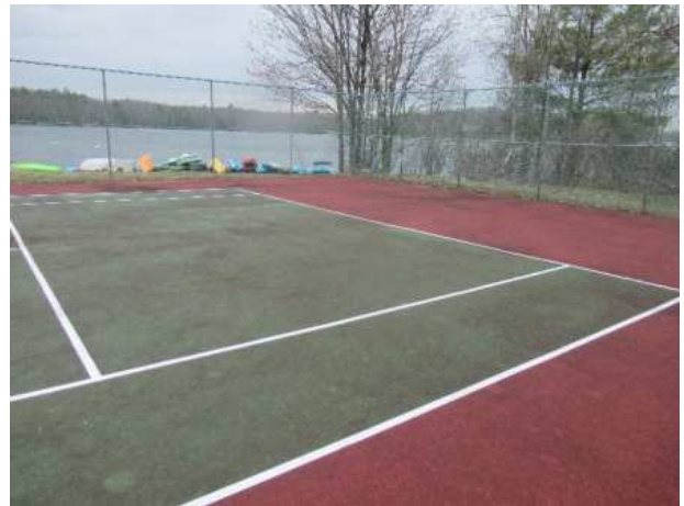
Stains at the tennis court at the pool house
