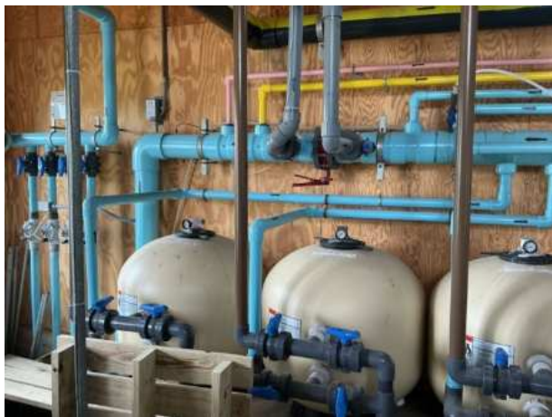
Pool mechanical equipment
