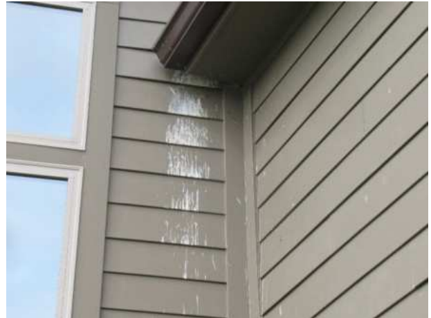
Stains at the entertainium building
