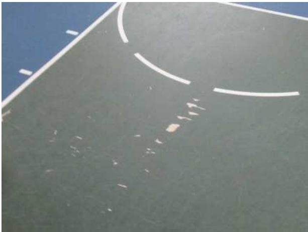
Scuffs and finish deterioration
