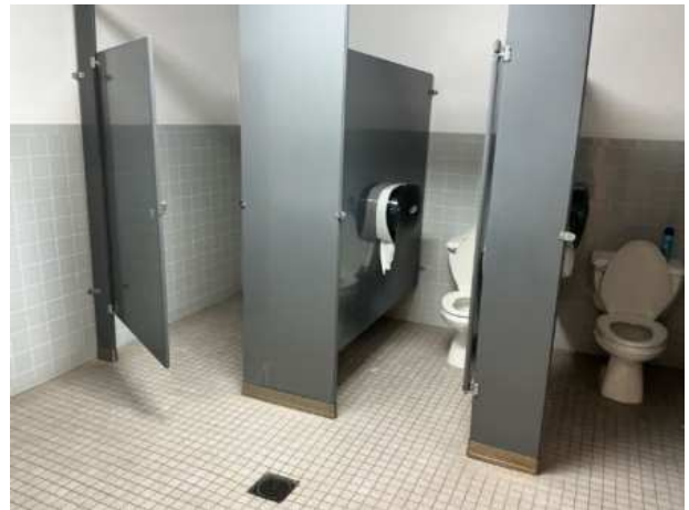
Rest room fixtures at the clubhouse
