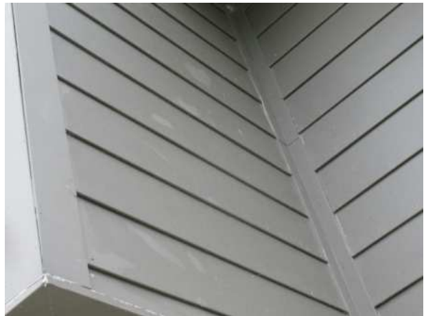
Paint finish deterioration at the pool house
