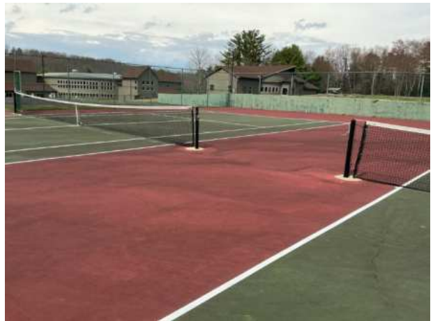
Stains at the Tennis court at the clubhouse
