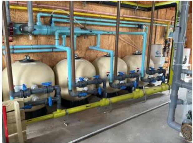
Pool mechanical equipment
