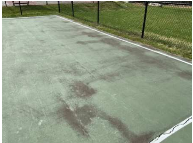
Stains at the basketball court
