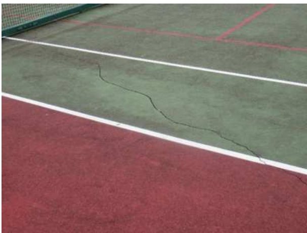
Cracks at the tennis court at the pool house
