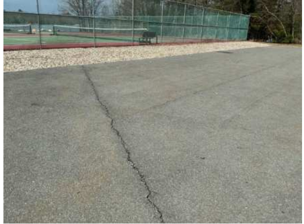
Cracks at the pool house parking area
