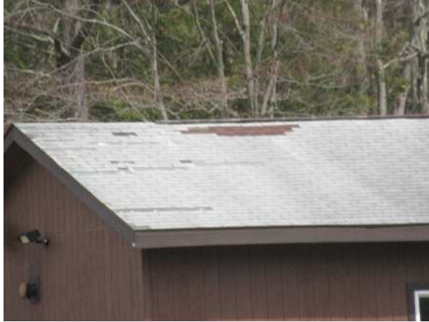
Previous replaced shingles, missing shingles and deterioration
