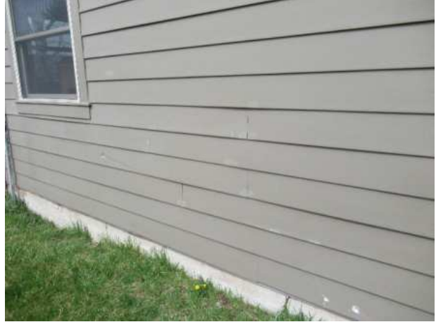
Paint finish deterioration at the clubhouse
