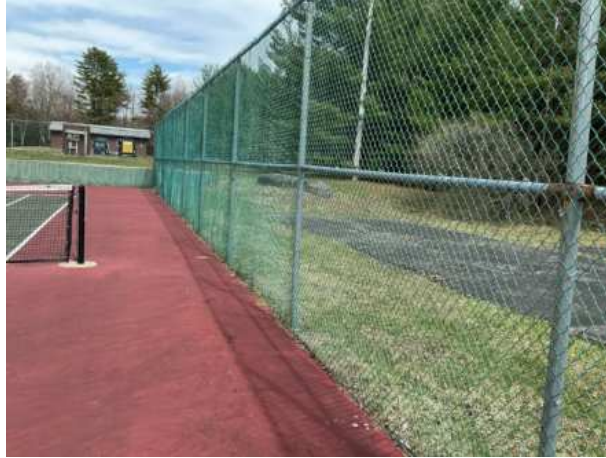
Tennis court fence at the clubhouse – note rust and warped webbing
