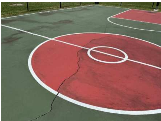
Stains and cracks at the basketball court
