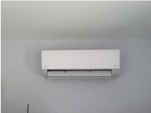
Mini-split air handling units at the pool house
