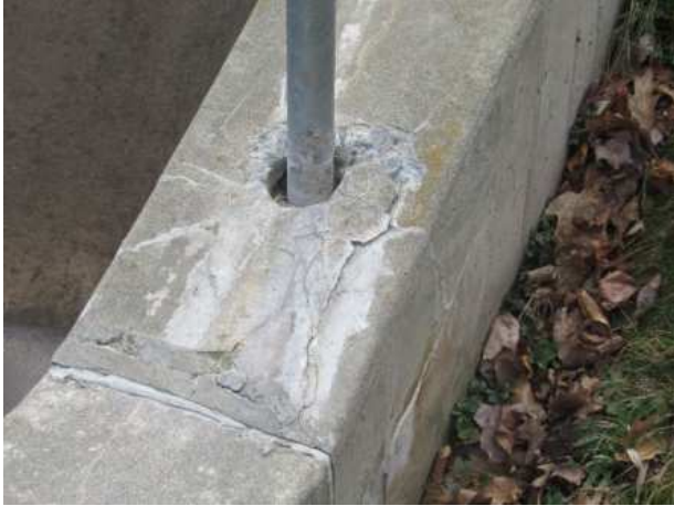
Cracked concrete at the railings
