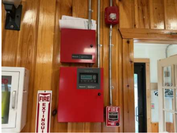
Control panel at the clubhouse
