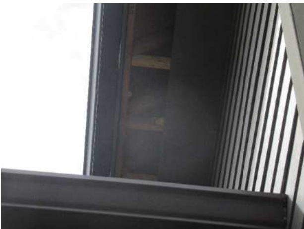
Missing soffit at the pool house
