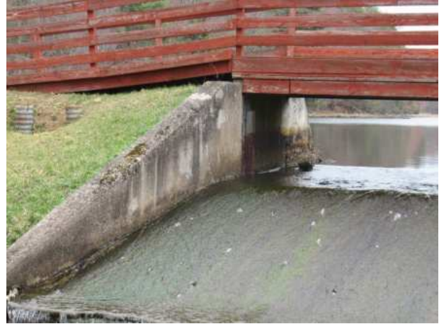
Concrete spillway at Lake Davies – Note concrete deterioration
