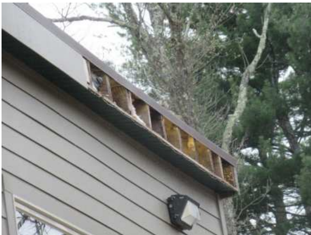
Missing fascia board at the entertainium building
