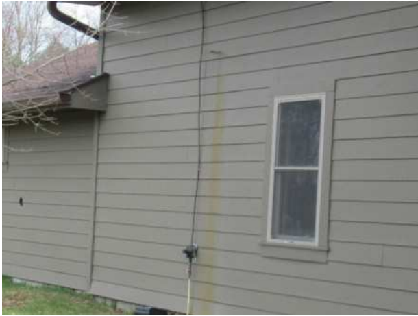
Stains at the clubhouse
