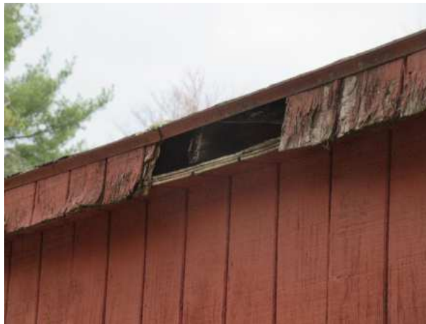
Missing wood trim
