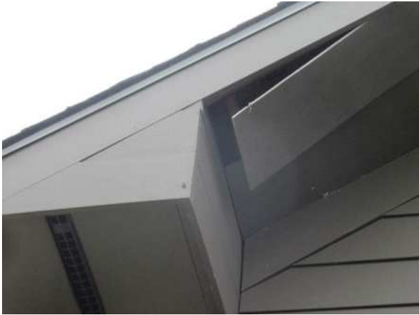
Loose soffit at the pool house
