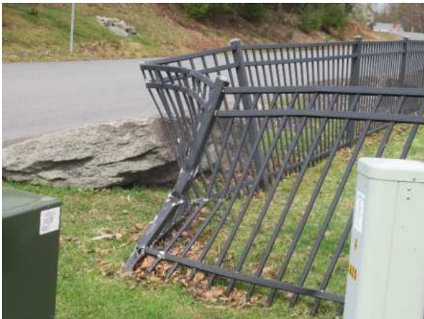
Fence damage due to vehicle collision
