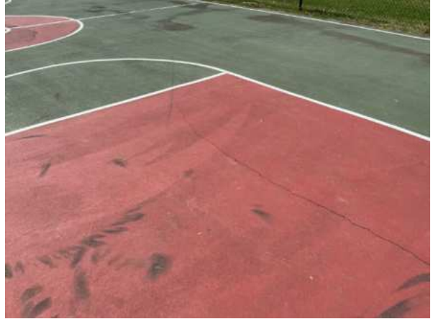
Cracks at the basketball court
