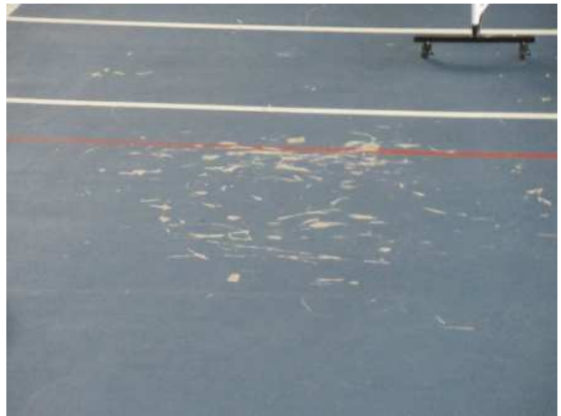
Scuffs and finish deterioration
