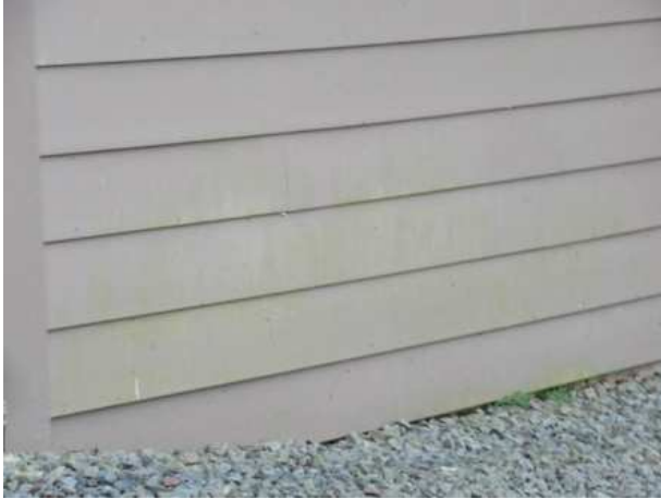
Stains at the entertainium building
