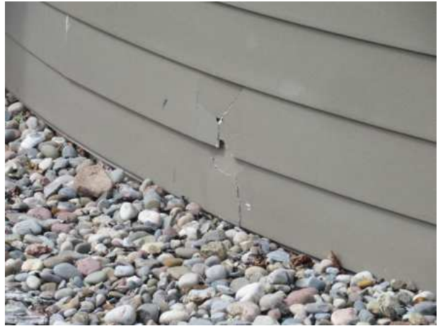
Damage at the clubhouse
