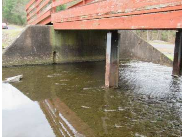
Rust at the metal columns
