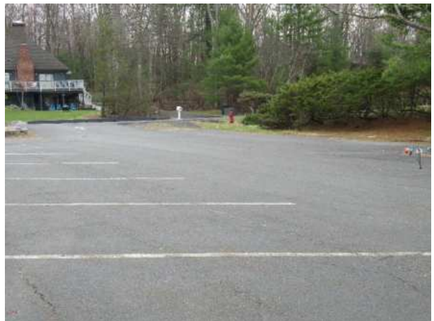
Cracks at the pool house parking area
