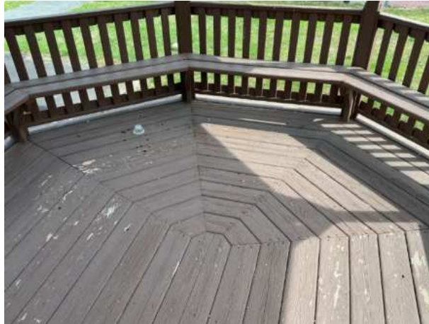
Wood deck boards – note deterioration
