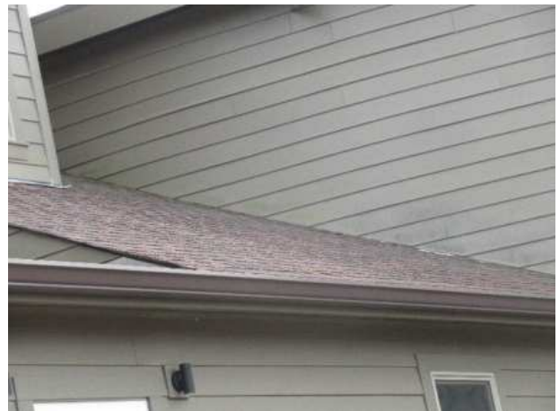
Stains at the entertainium building
