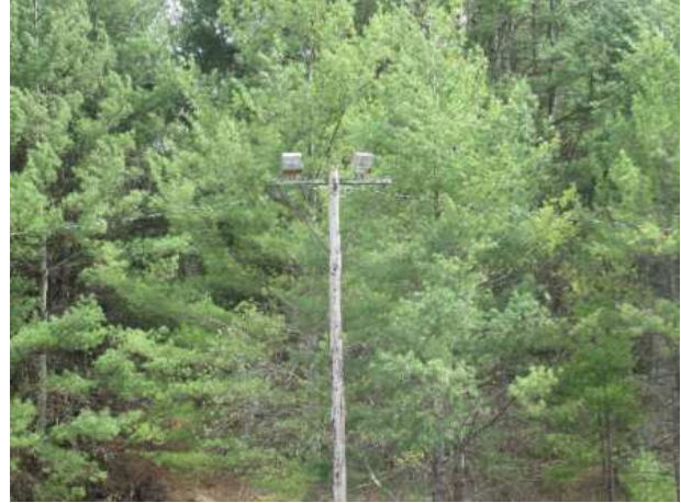
Light pole and fixtures at the upper lot by the clubhouse
