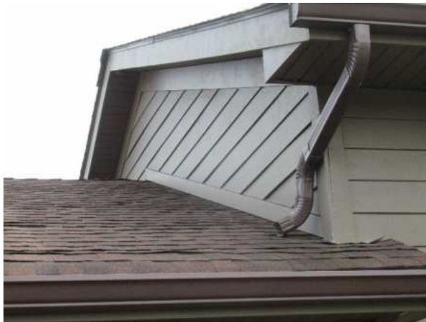
Shingle lift and downspouts discharge directly onto lower roof at the clubhouse
