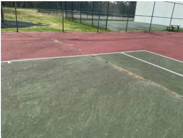
Cracks at the Tennis court at the clubhouse
