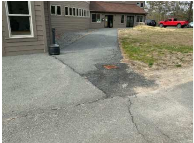
Cracks and deterioration
