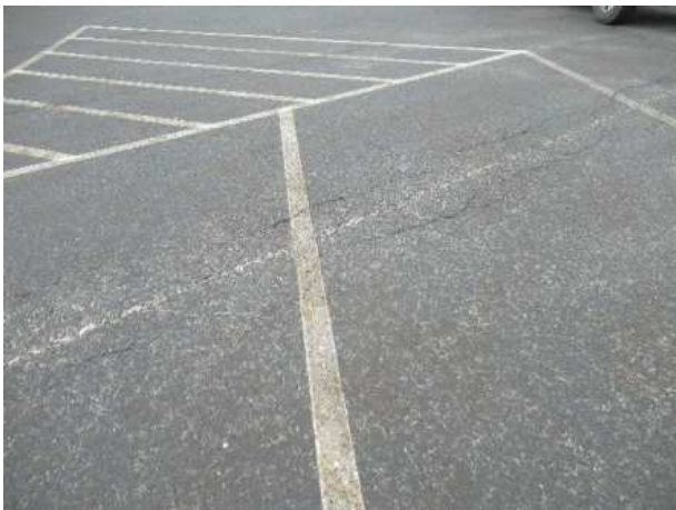
Cracks at the pool house parking area
