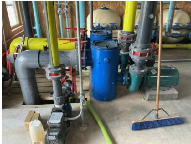
Pool mechanical equipment
