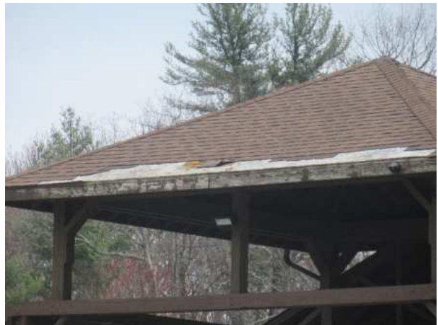
Missing shingles and deterioration
