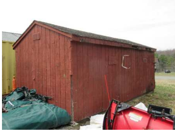
Wood damage and deterioration
