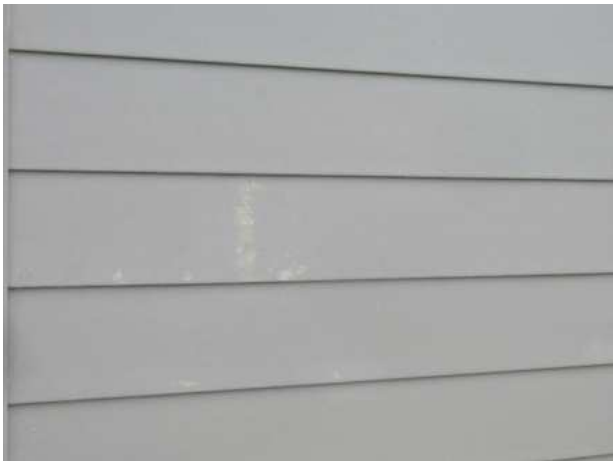
Paint finish deterioration at the pool house
