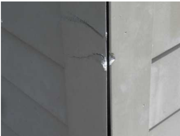
Damage at the pool mechanical building
