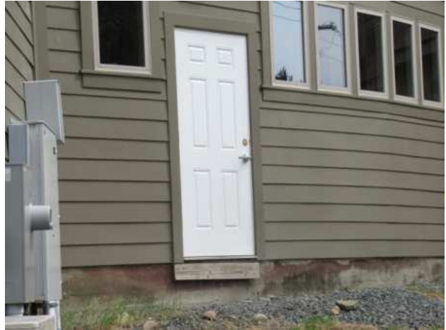
Doors - We note door exits are not at grade
