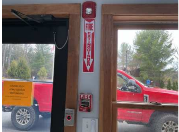
Emergency devices at the clubhouse
