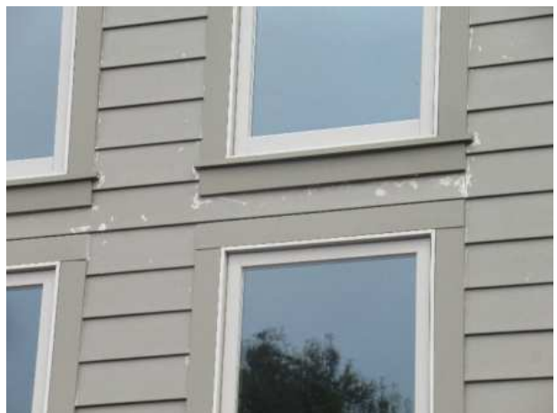
Paint finish deterioration at the pool house
