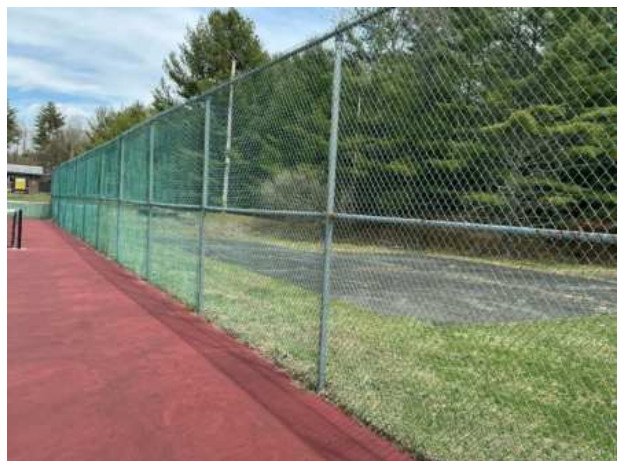
Tennis court fence at the clubhouse – Note warped webbing
