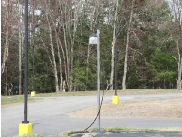
Light pole and fixture at the upper lot by the clubhouse
