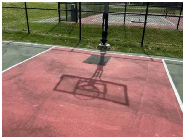
Stains and color coat deterioration at the basketball court
