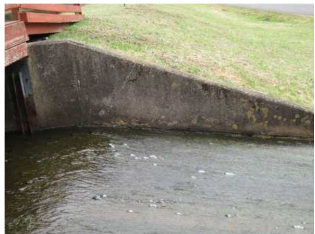
Concrete spillway at Lake Davies Note concrete deterioration and cracks
