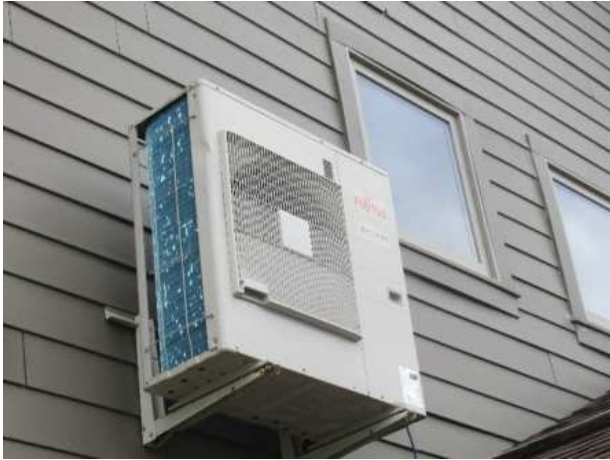
Mini-split condensing units at the pool house
