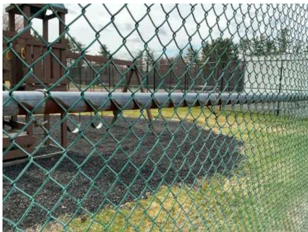
Tennis court fence at the clubhouse – note rust
