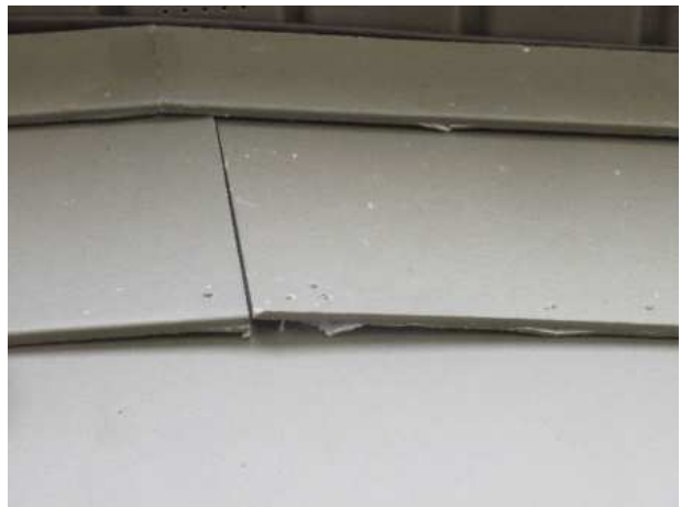
Loose siding at the clubhouse
