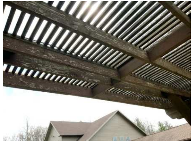
Weathered wood and finish deterioration
