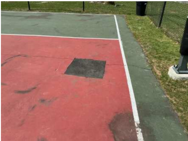
Patch repair and cracks at the basketball court
