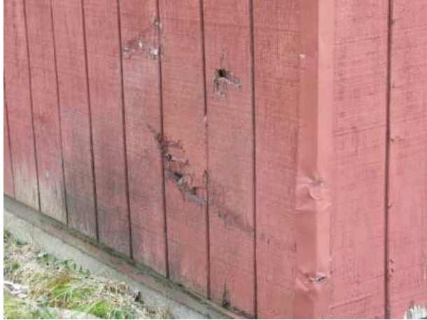
Wood damage and deterioration
