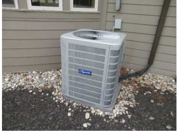
Condensing unit at the clubhouse
