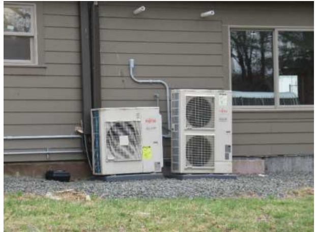
Mini-split condensing units at the Entertainium building
