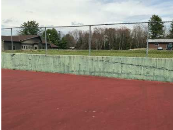
Cracks and deterioration
