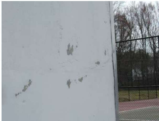
Cracks and finish deterioration
