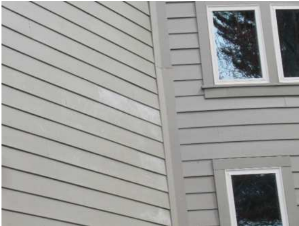
Paint finish deterioration at the entertainium building
