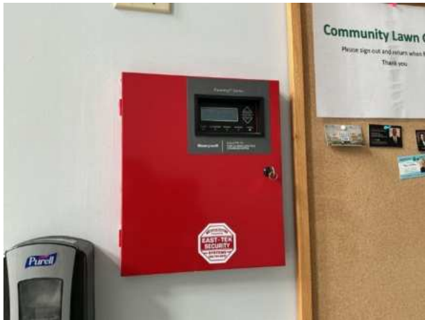
Control panel at the pool house
