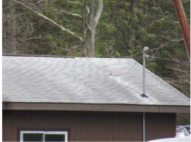
Stains and weathered shingles
