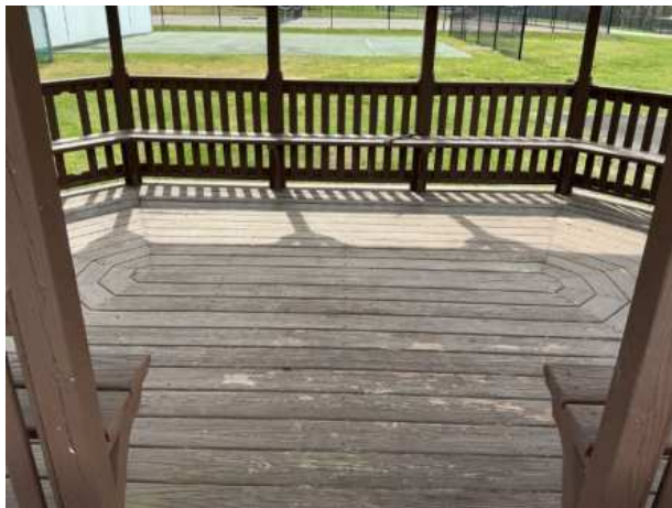
Wood deck boards – note deterioration
