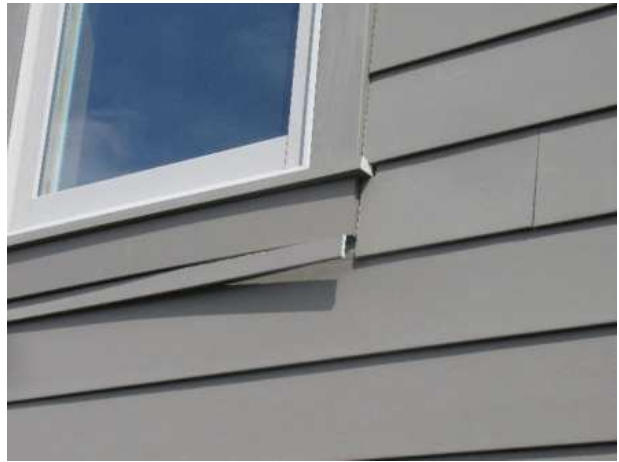
Loose trim at the pool mechanical building
