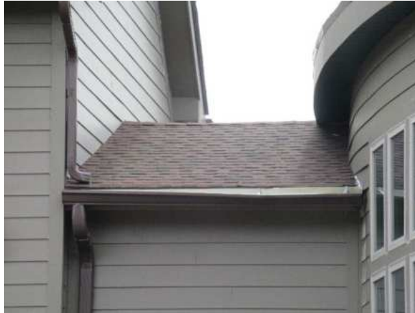
Downspouts discharge directly onto lower roof at the entertainium building
