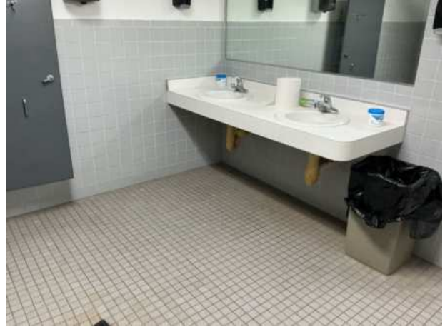
Rest room fixtures at the clubhouse
