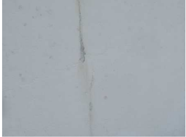
Cracks and finish deterioration
