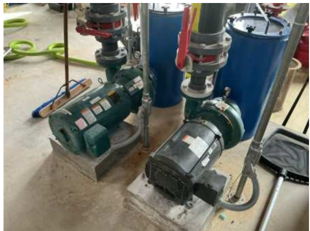
Pool mechanical equipment
