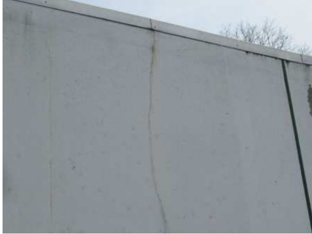
Cracks and finish deterioration
