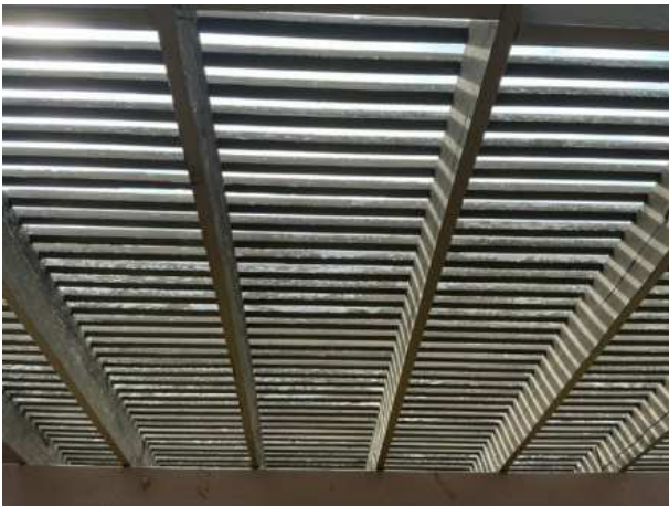
Paint finish deterioration
