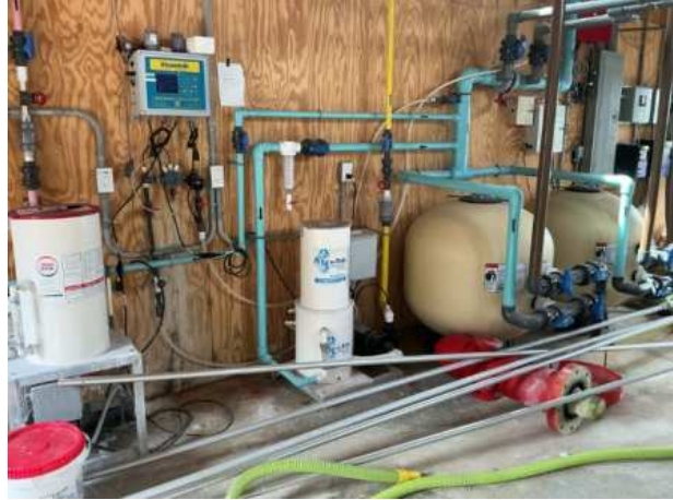
Pool mechanical equipment
